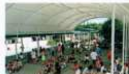
School covered playground - 1994 New Zealand - Précontraint® 702 Tensile resistance after 14 years: Warp 96% - Weft 98%
